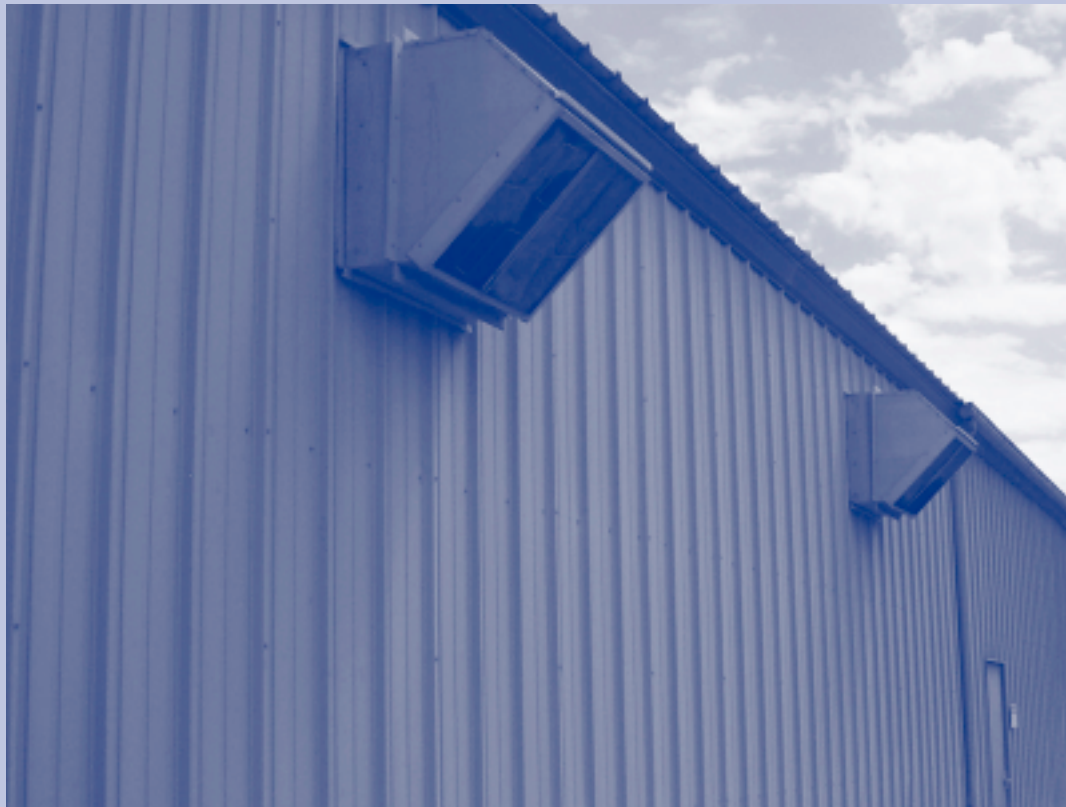
Ventilation Filters on Compressor Room Filter Wall
